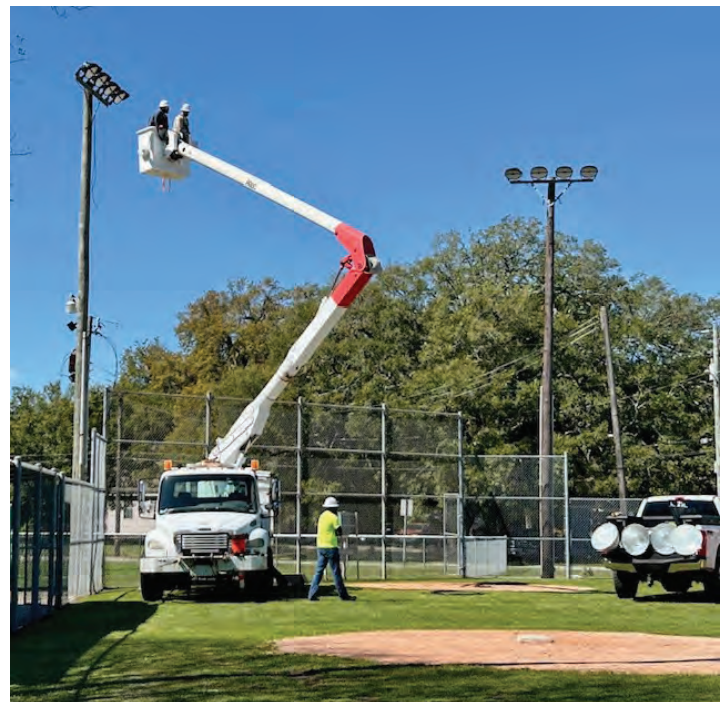
▲ New LED lighting added to Savarro Park
