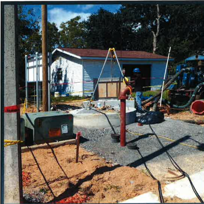
NOB5- Michelle Drive Pump Station
