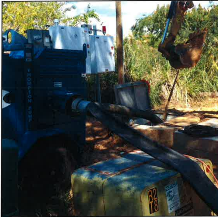
NOB4- Bayside West Pump Station
