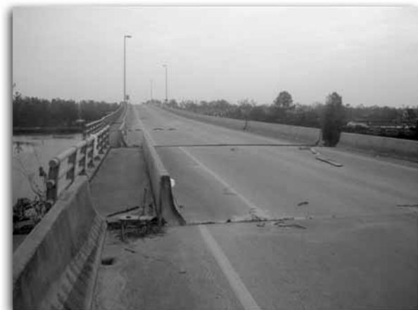
Katrina's fury shifted sections of the north end of Popp's Ferry bridge.
