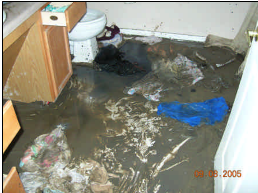
Another Hope VI unit. All units in the Hope VI project took at least five feet of water. Many were flooded to the second floor.
