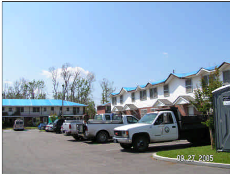
The roofs were covered immediately to mitigate further damage. With proper funding, this site named Fernwood can be put back in full repair quickly.
