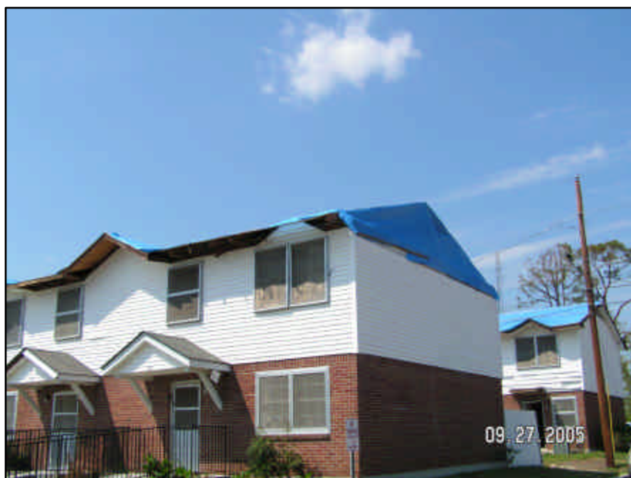
The roof was completely blown off on the right end of the building. The two end units' upper and lower floors took heavy water damage that intruded into the other units as well.
