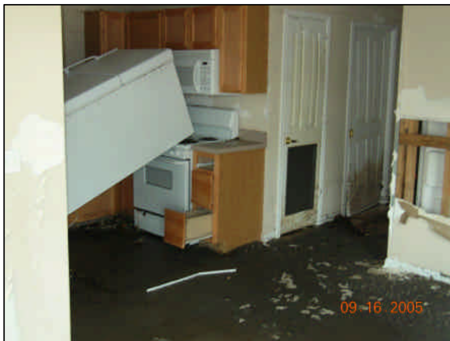
Another kitchen in Hope VI. The vinyl composite flooring is covered in both Back Bay mud and Keegan Bayou wastewater treatment sludge.
