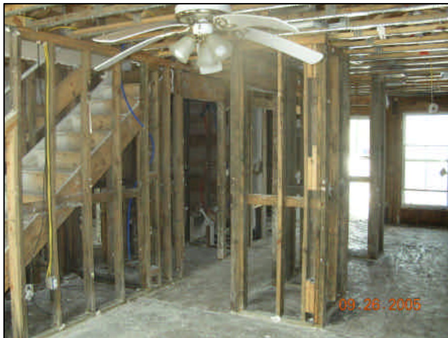
A HOPE VI unit after gutting the wet drywall, carpet, cabinets, appliances, and other items. This unit can be saved since the authority took quick action. The upstairs portion is in good shape. All that's needed now is funding to put it back together.
