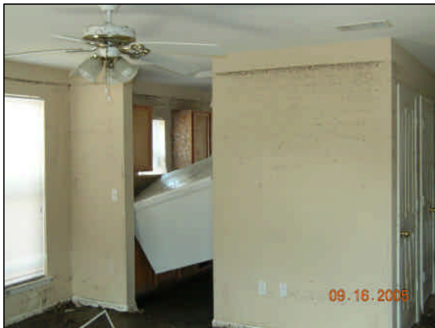
Over seven feet of water in this HOPE VI unit. Notice the refrigerator that is jammed between the walls after it floated out of place.
