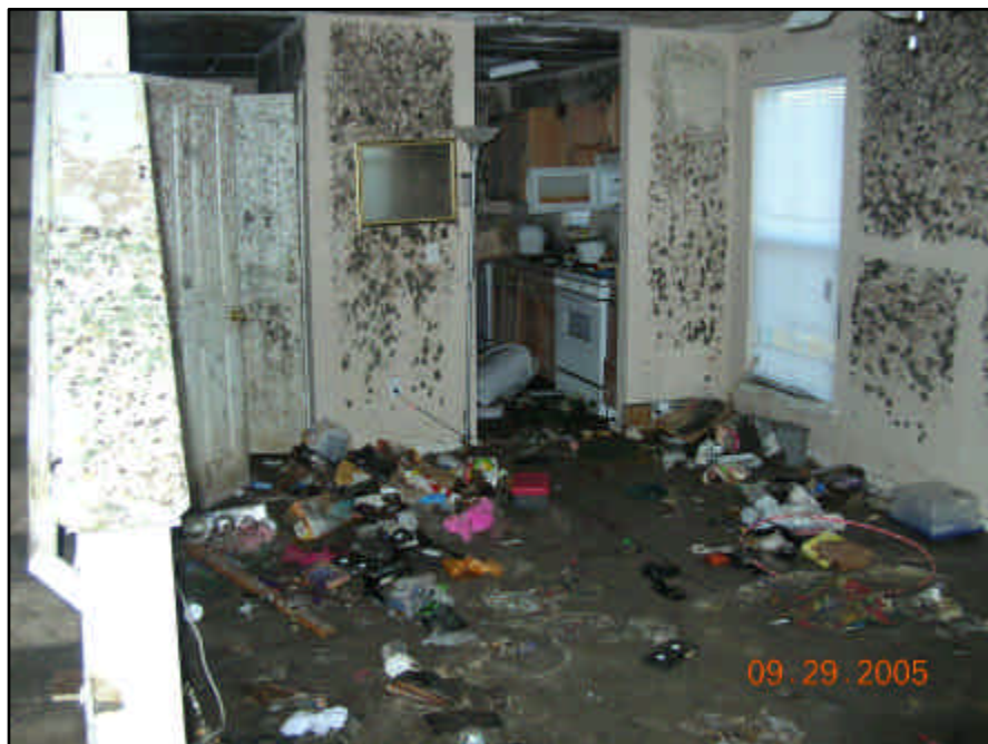
This unit took water to the ceiling. The mold and sludge in this unit is typical of most of the HOPE VI units. The debris was washed into the unit
