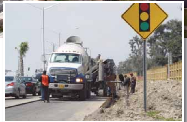
MDOT contractors install new curbing, part of the total remake of Beach Boulevard.
