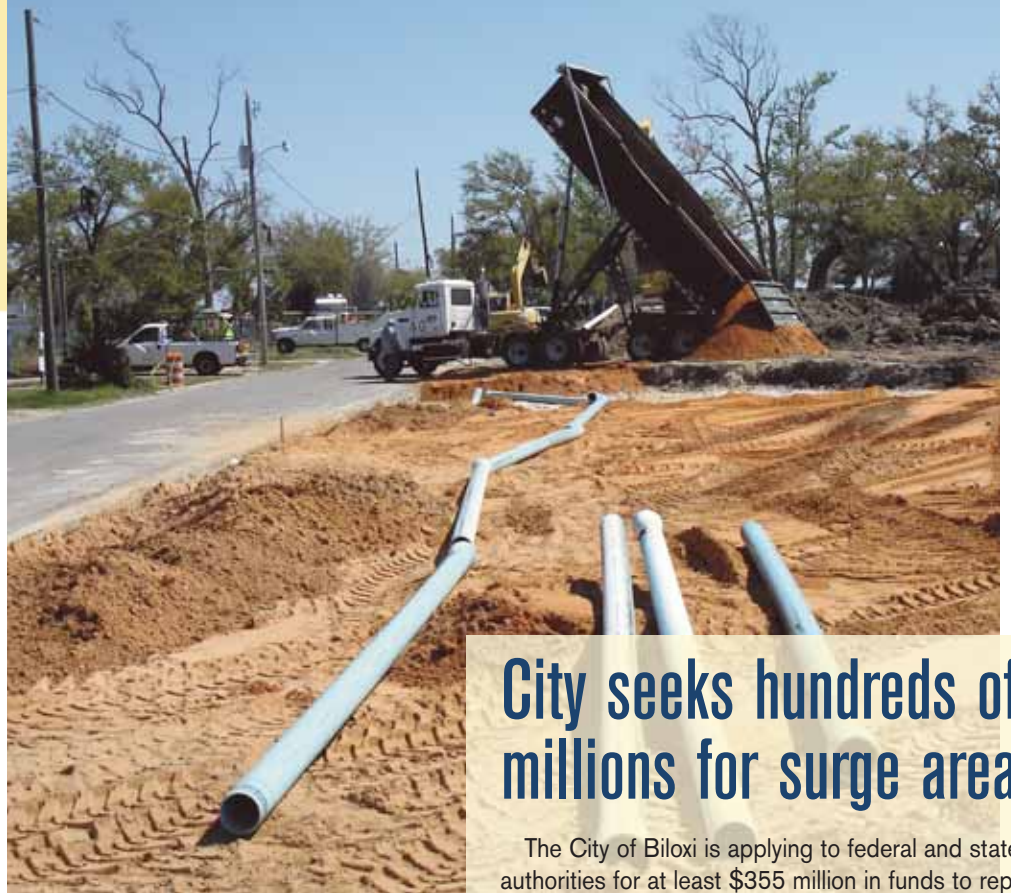
The city of Biloxi is planning hundreds of dollars in infrastructure work, primarily in storm-surge areas of the peninsula and the Eagle Point area. Here, Public Works crews install a new water line on Kensington Drive on Back Bay.
